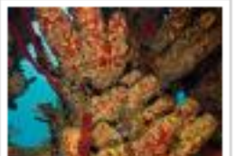
The pilings of the pier are overgrown with marine life.
